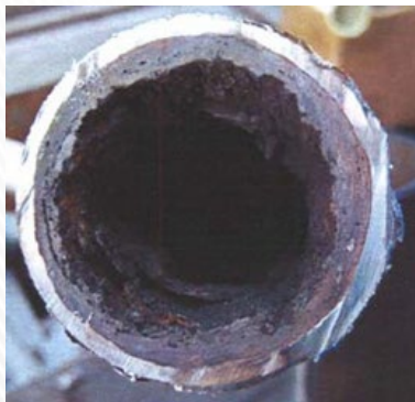
Bore reduction by corrosion.
