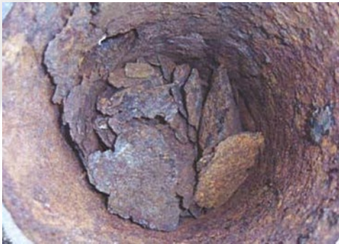
Bore reduction by corrosion.
