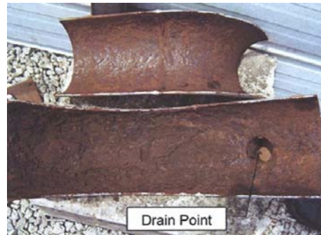
Thinning of Wall Section.
