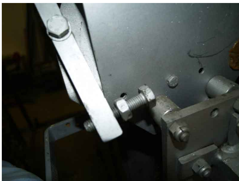
Rocker arm with adjusting bolt - Note: bolt is not locked
