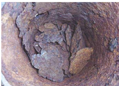
Blockage in 6” elbow.
