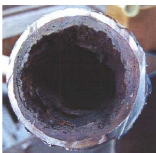
Bore reduction by corrosion.
