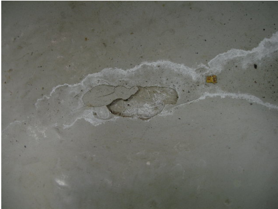
Picture 1 - Chemical attack causing blisters
