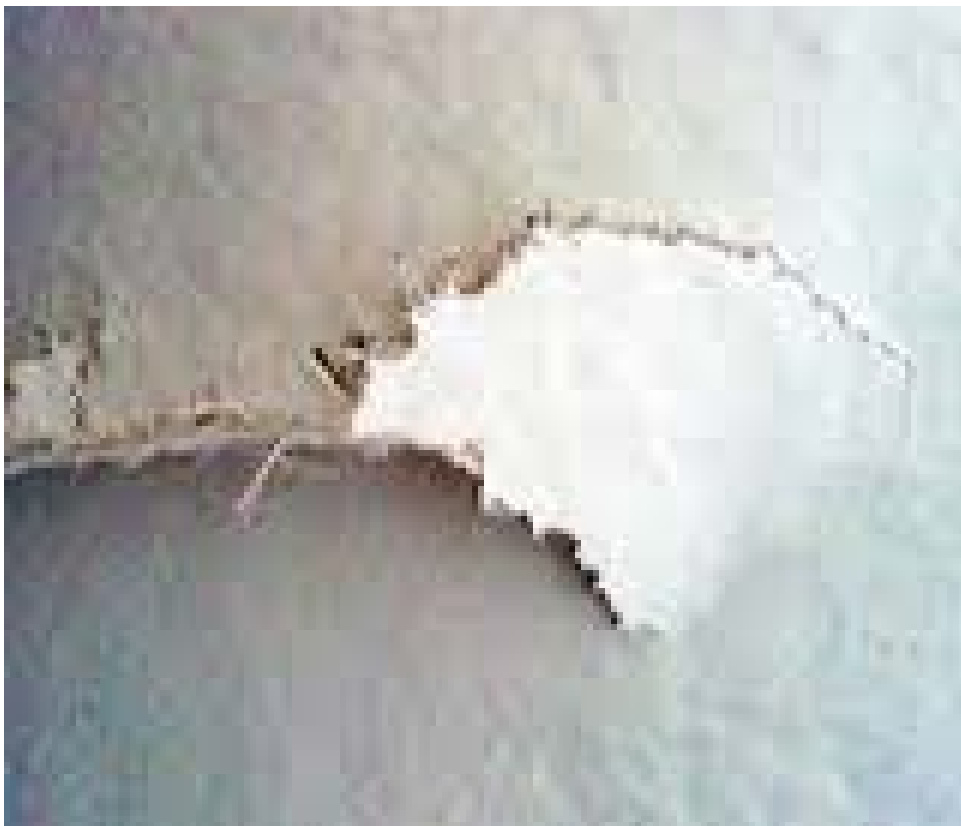
Picture 4 - Poor bonding at manufacture
