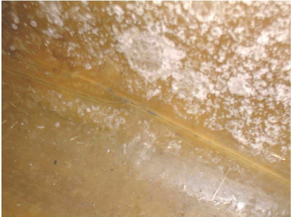
Picture 5 - Crack propagating from base to shell attachment.
