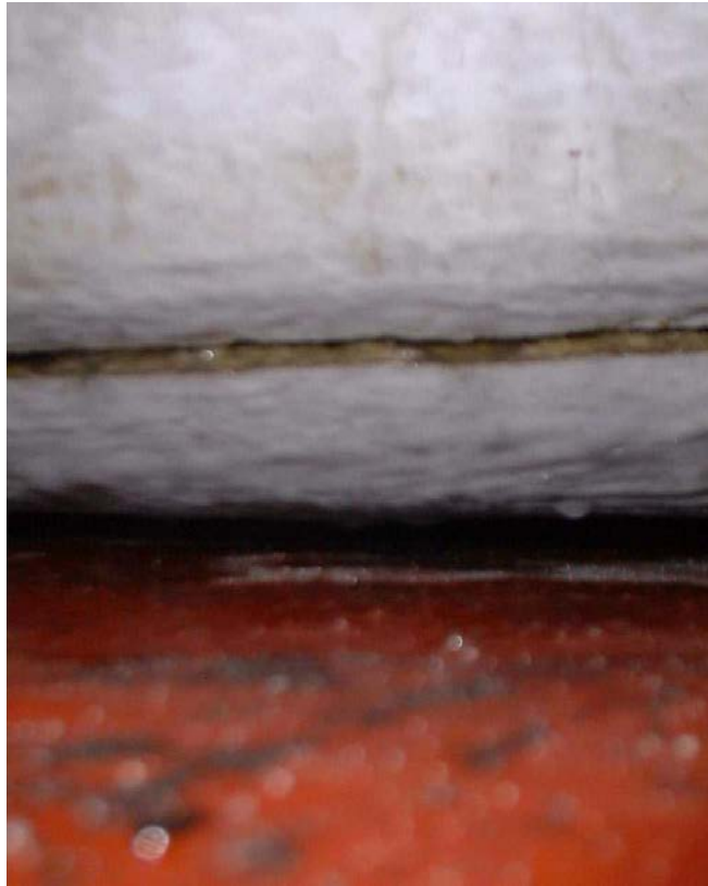
Picture 7 - Insufficient landing on base causing excessive load leading to cracking
