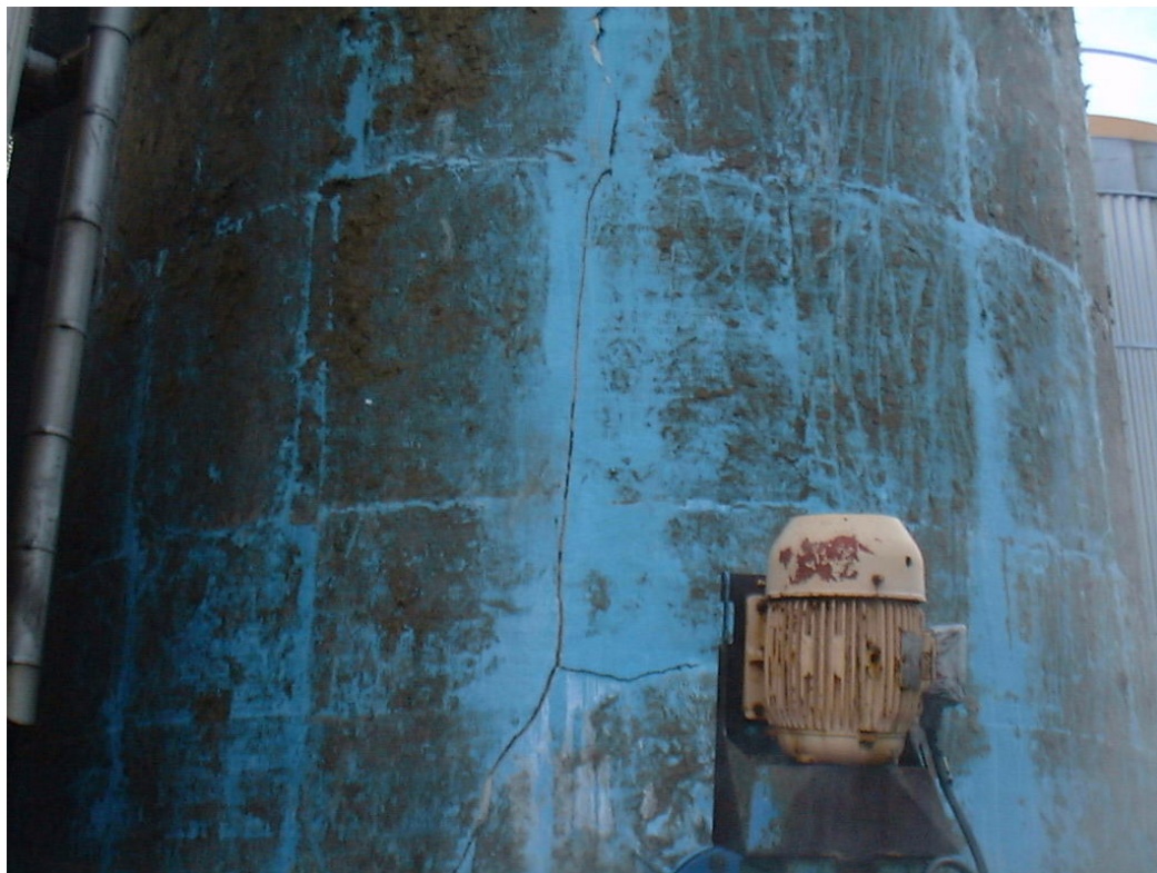
Picture 8 - Severe cracking on shell
