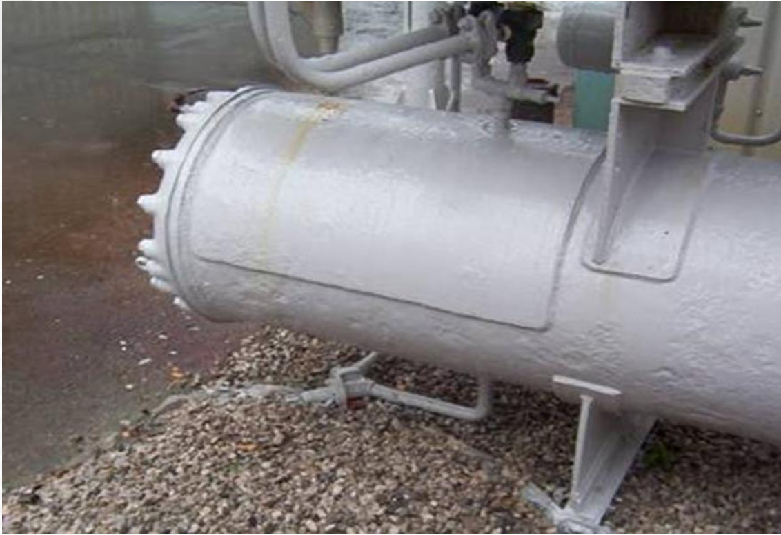
Use of a fillet welded temporary repair over corroded region of heat exchanger
