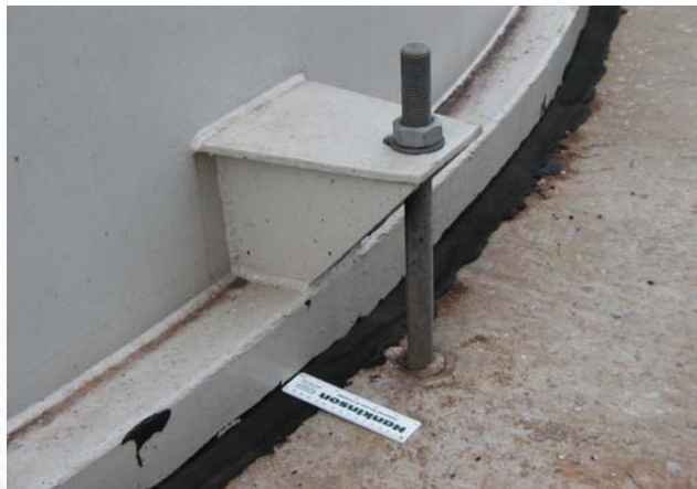
Example of external floor plate lifting from the foundation
