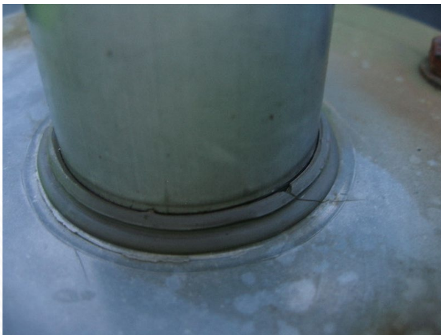
Picture 6 - Environmental Stress Cracking (ESC)
