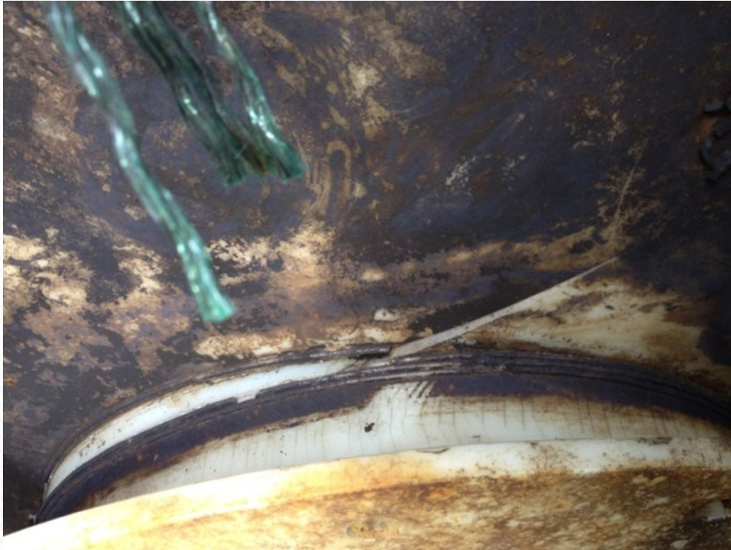
Picture 3 - Environmental Stress Cracking (ESC) horizontal cracks with through wall cracking
